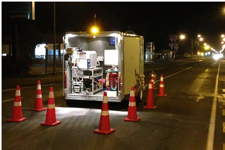
The DWS team worked day and night to complete these works on time.
